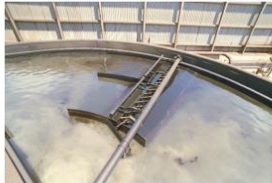
Wastewater treatment plant (Tenerife site).
